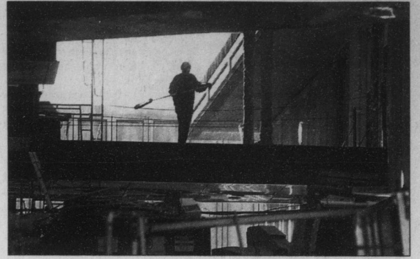
DTH/JESSICA NEWFIELD A construction worker at the Student Union sweeps a walkway between the existing building and the new addition.
