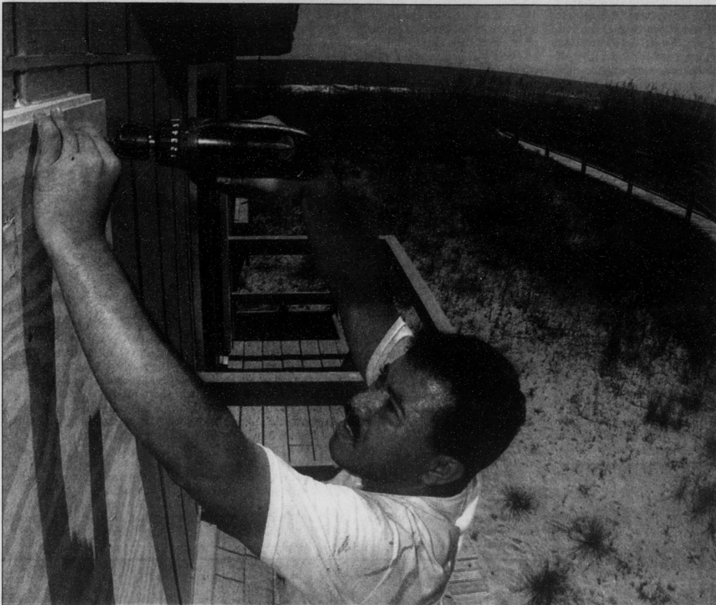
Ramone Santiago of Kerwick Painting Service covers the window of an oceanfront house with plywood on Monday at Carolina Beach. Kerwick Painting Service also has been contracted to prepare condominium units for Hurricane Isabel, which is expected to hit the coast Thursday.
