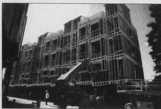
Construction on Rosemary Village continues on West Rosemary Street near Mama Dip's restaurant. The complex will be ready by December.
