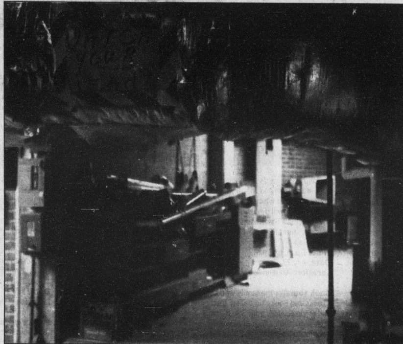
The hallway leading to "the cage" also exposes the building's plumbing — students taller than about 5 feet have to duck to get through, but they can find plenty of seemingly random scrap material.
