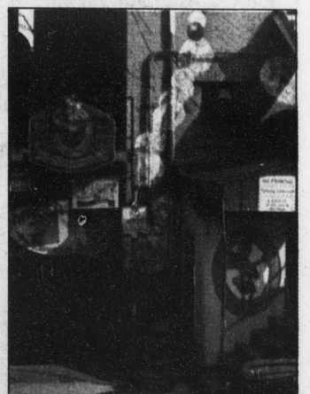
The Rathskeller restaurant is closed for repairs, but it is expected to be open by the time students arrive back for school.
