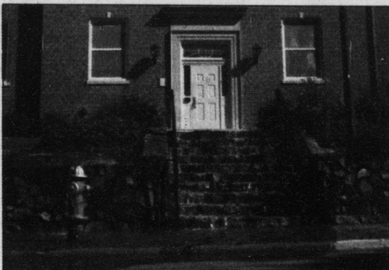
The steps to Joyner Hall spill over with water Wednesday after a relief valve malfunctions, leaving several dorms without heat for two hours. DTH/PAUL KIERNAN
