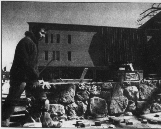
Javier Barilla works on brickwork outside of the University's new FedEx Global Education Center, which has faced two and a half months of delay.
