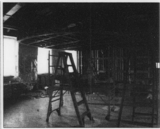
Construction continues on the Starbucks replacing End Zone in Rams Head. If materials arrive on time, the facility should open in late April. DTH/CASSIE BUTLER
