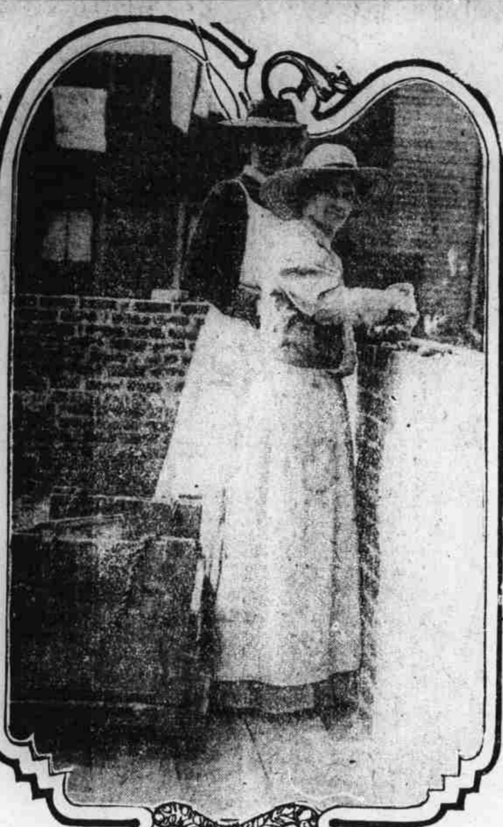
Sisters Anna and Daisy of the Apostolic Church in Jersey City, laying bricks of the new church which they and ten other women (three children and five men) are erecting without cost for labor. The edifice in the ordinary course of construction would cost $40,000. It will be completed some time in November. "Mother" Sarah B. Earl founded the congregation of the sect in Jersey City seventeen years ago. She has many followers and all have undertaken to fetch and carry and dig and delve and mix, without recompense, so that the church may be built.
