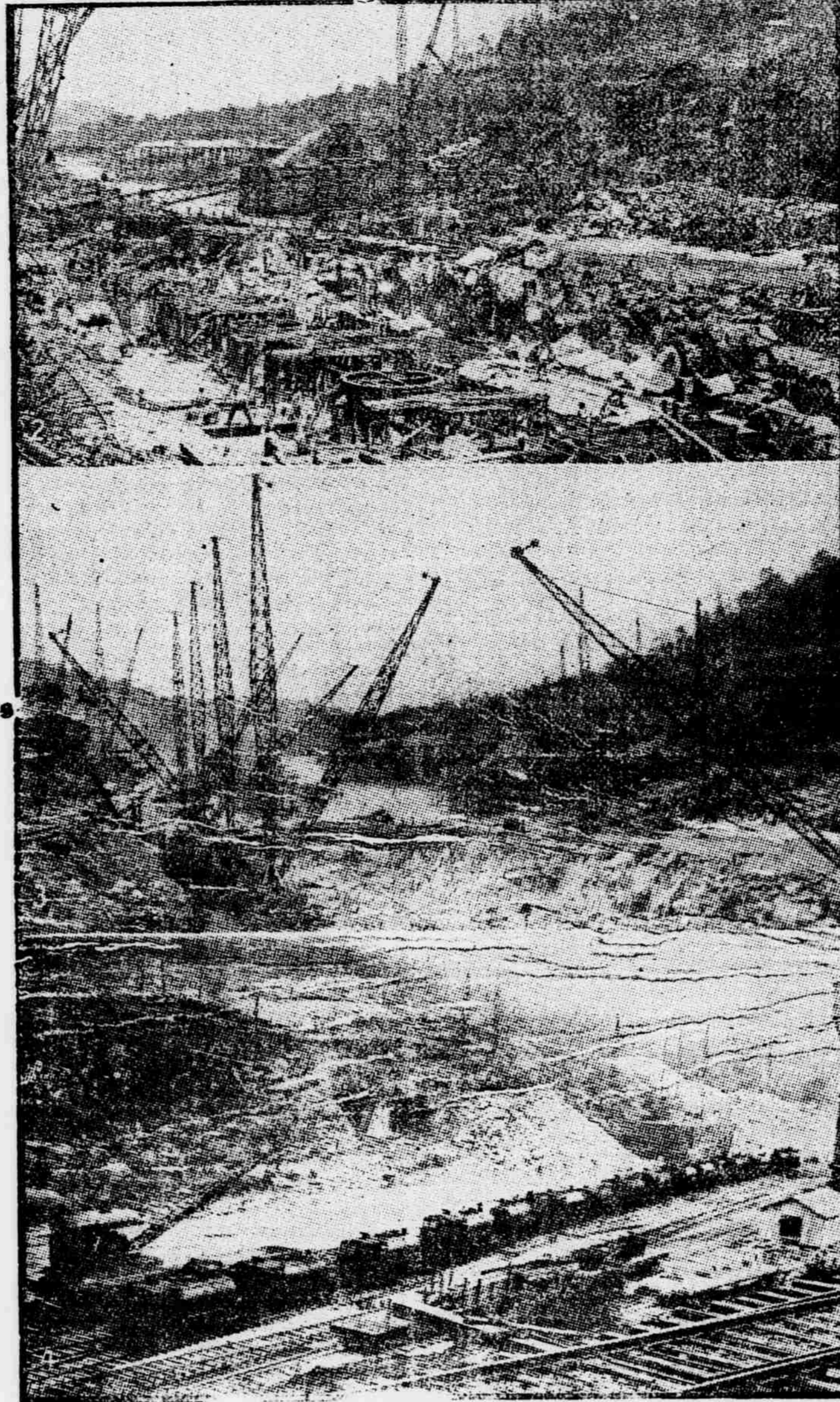
DEVELOPMENT BY ALUMIUM COMPANY OF AMERICA AT BADIN, N.C. 1—Excavation for power-house. 2—Forest of derricks at work in gorge. 3—Saddle-tank locomotives with upper portal of tunnel.
