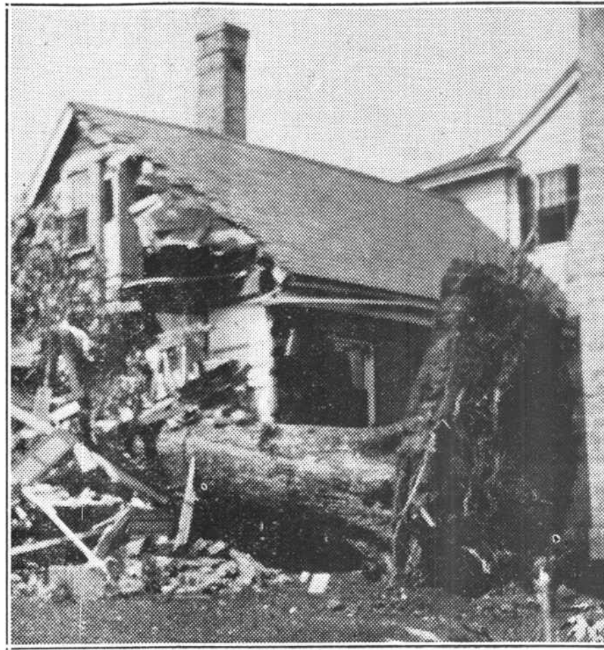
Uprooting of giant oak tree by high wind of Sunday afternoon causes heavy damage to kitchen wing of Mrs. A. E. Jones' home in South Warrenton. Hundreds of persons following the storm visited this scene.
