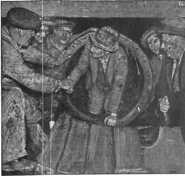
Hundreds of feet below the waters of the Hudson the north tube of the Lincoln Vehicular Tunnel is "holed through" to connect New York and New Jersey. The tunnel is designed with two tubes, each one-way. The south tube is already in use. The north one will be completed next year. As a climax to the two-year digging job, sand-hog crews from each shore meet near center of the river bed.
