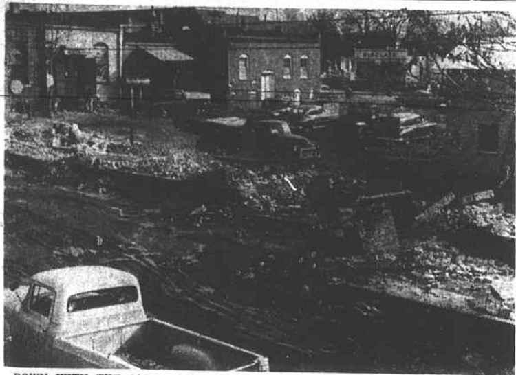
DOWN WITH THE OLD — Debris from the old storage houses back of the Warrenton Department Store is shown as the lot is being cleared for a parking lot. W. L. Wood, chairman of the Street Committee of the town, told the commissioners at their meeting on Monday night that Mrs. W. H. Hughes, Jr. of Raleigh, owner of the building, had agreed to lease the lot to the town as a parking lot. He said that adjoining property would also be graded, and that it is hoped that the lot would be ready for use by March 1. Committee reports and other routine matters occupied the attention of the commissioners during their unusually brief session Monday night. (Staff Photo)
