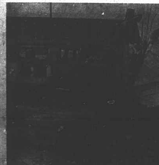
MAKING WAY FOR NORLINA POSTOFFICE—A bulldozer topples a wall of the Old Community Motor Service building at Norlina to make room for the new post office which is expected to be ready for occupancy by July 1. The building gutted by fire several years ago, will be demolished and the lot leveled before construction of the new post office begins in the next few days. (Staff Photo)
