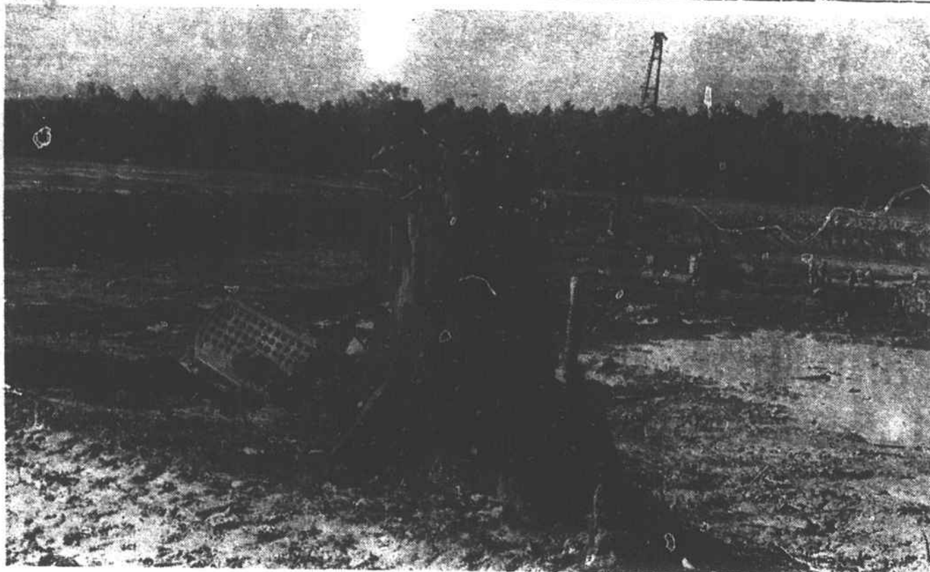
Once a majestic sentinel on the Roanoke River near Eaton's Ferry, a shattered tree stump awaits removal as men and machines clear area for a new bridge which will span the Gaston reservoir. The bridge will replace the ferry now in
