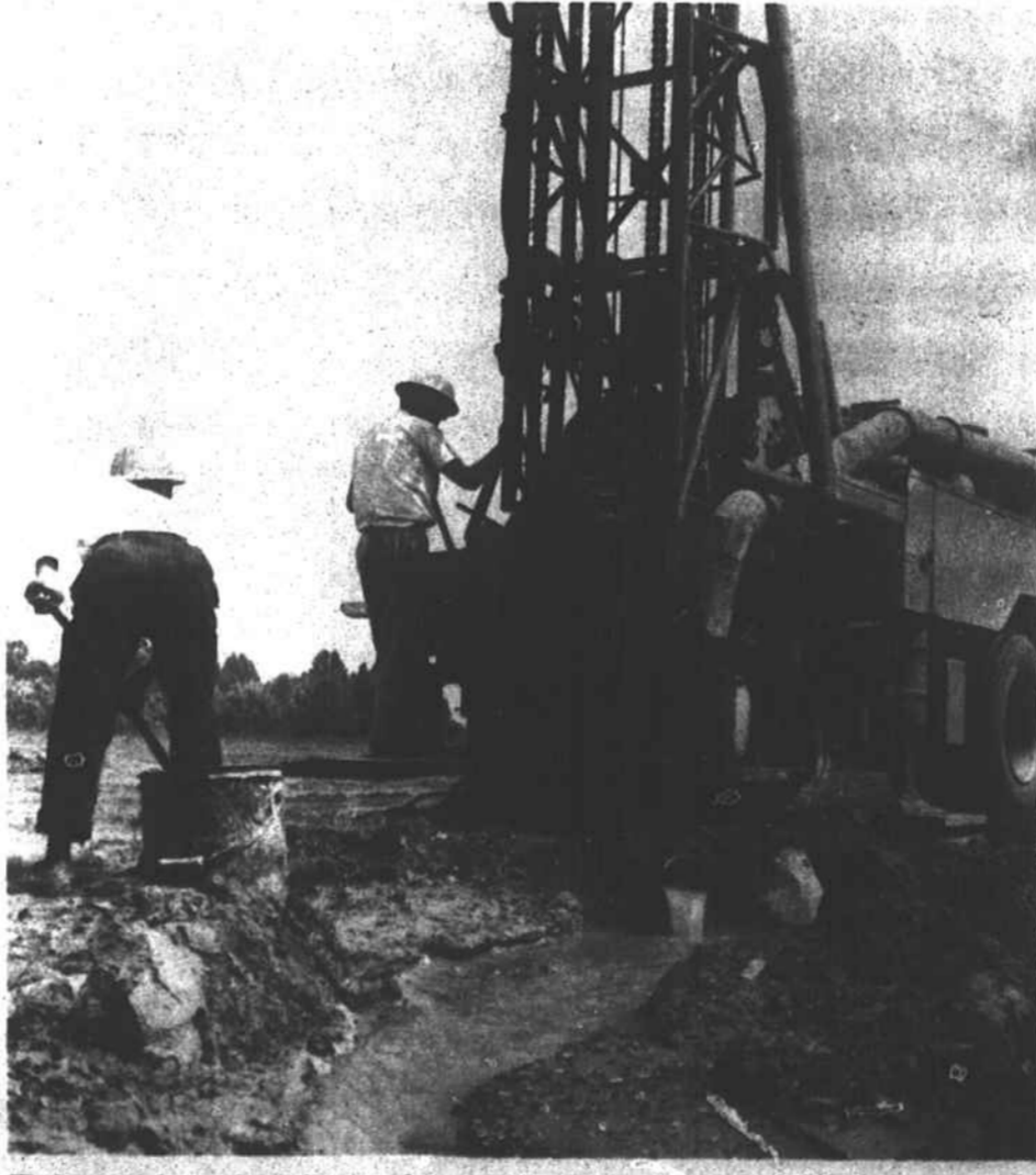
Workmen sink a well at the site of a new Negro elementary school in southern Warren County. The well, completed over the weekend, paves the way for the construction of the new building which will serve Negro
