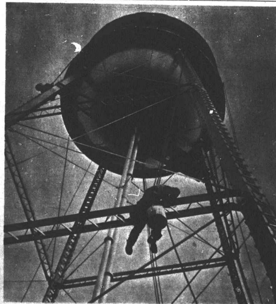
The Warrenton water tank is undergoing a periodic painting. The high perched painter was caught by the camera of photographer Bill Jones on Tuesday.
