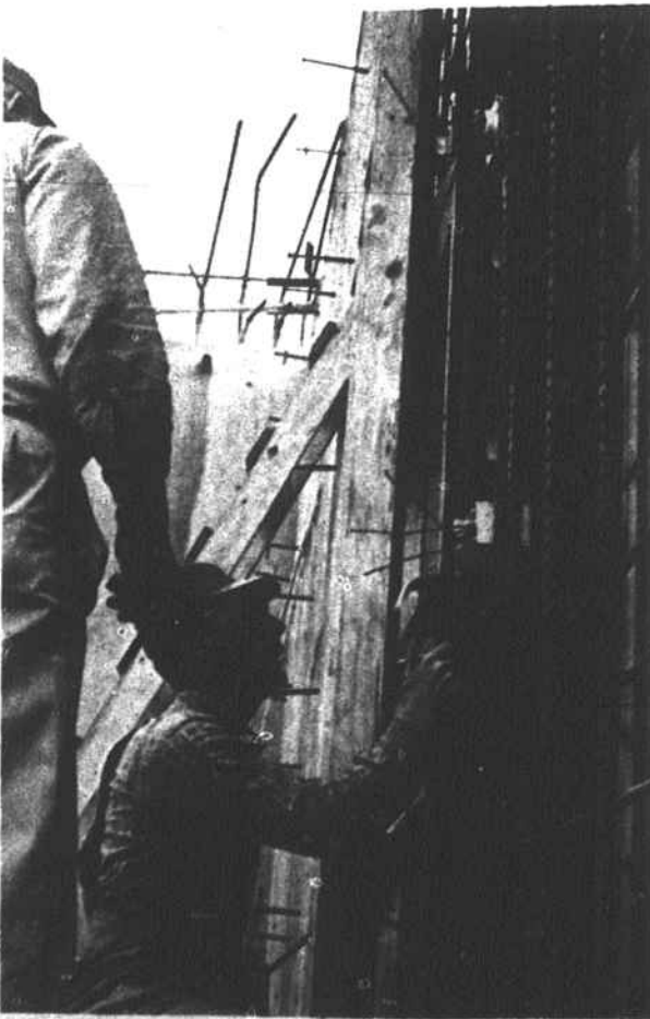
Workmen are shown constructing a telephone tower at Afton this week. The tower is one in a link of towers being built by the Bell Telephone Company. A temporary tower was erected on the site for testing purposes several months ago.
