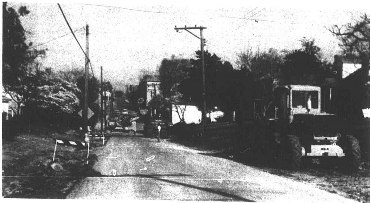
Work has started on the widening of Franklin Street at Warrenton. The scene shown above is between White's Gin and Hawkins High School. Harold R. Skillman, superintendent of the Warrenton Water Company, said that he anticipates that it will take about two months to finish the project.
