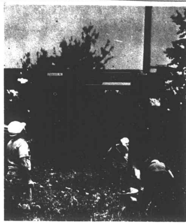
An extra crew from Stackhouse, Inc., is working in the Enterprise Community to speed up construction of heavier lines in the Lake Gaston area.
