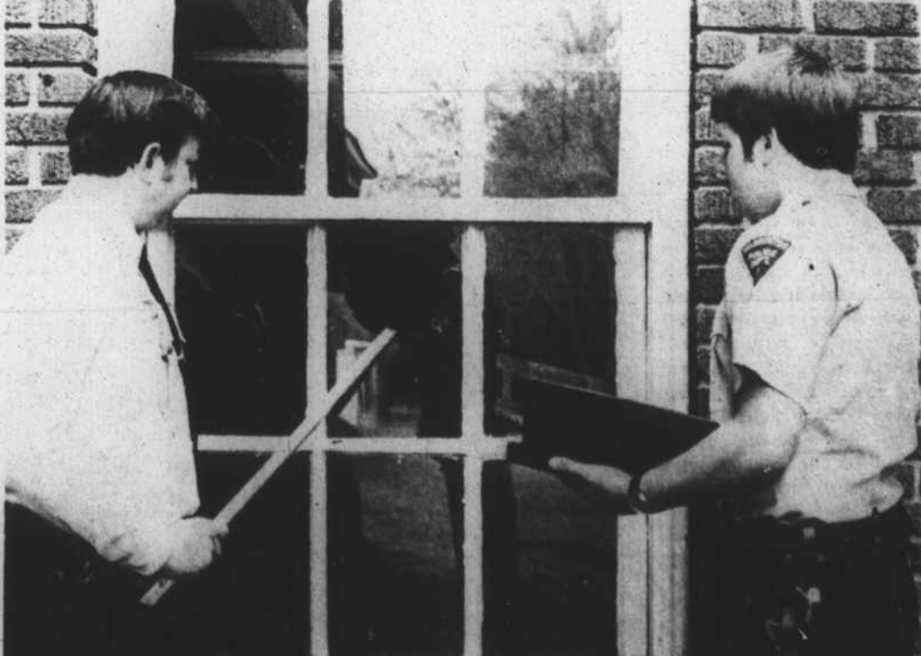
Warrenton Police Chief Freddie Robinson (left) and Officer Bobby Bolton examine a broken window that was believed to have been the point of entry in a weekend break-in at John Graham High School. Chief Robinson said investigation of the break-in is continuing. [Staff Photo]
