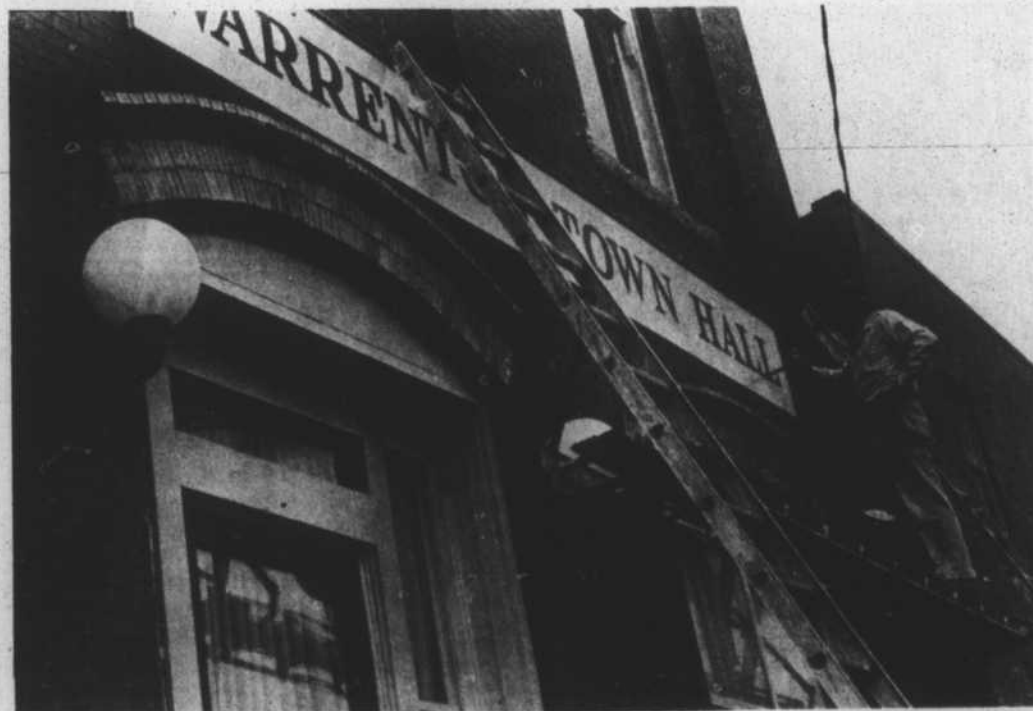
FINISHING TOUCHES—Bobby O. Burnette, Henderson sign painter, completes the lettering on a new sign gracing the recently remodelled Warrenton Town Hall. As the sign was completed last week, town employees began painting over an old Boyd-Boyce Motor Co. sign on the wall of a downtown store, and firemen oversaw the burning of the remains of the old Baptist Church on South Main Street Tuesday night in other beautification efforts. The church foundation will be levelled by bulldozer enabling workers to keep the area clear of undergrowth. (Staff Photo)
