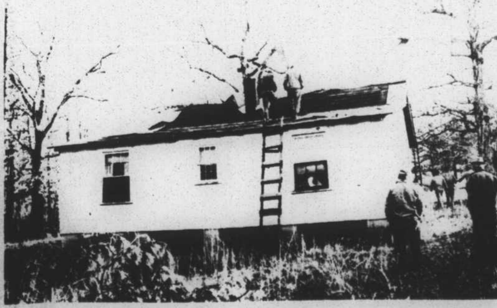
Most heavily damaged during Monday afternoon's high winds was the home of William Short in the Embro community. The roofing was ripped off and windows smashed in the dwelling. Short was not at home at the time.
