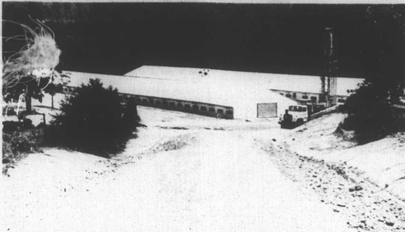
These two long chicken houses are being erected near Warren Plains by Macon Myrick of Norlina. The houses are part of early development of Perdue Farms' Warren County operation, centered on a 500-
