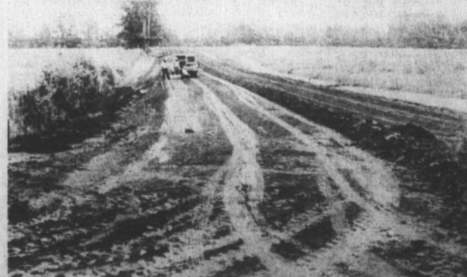
Workmen are shown on Tuesday morning constructing an access road to the site of a PCB storage landfill at Afton. Settlement of a suit by Warren County last week led to the beginning of construction. (Staff Photo)
