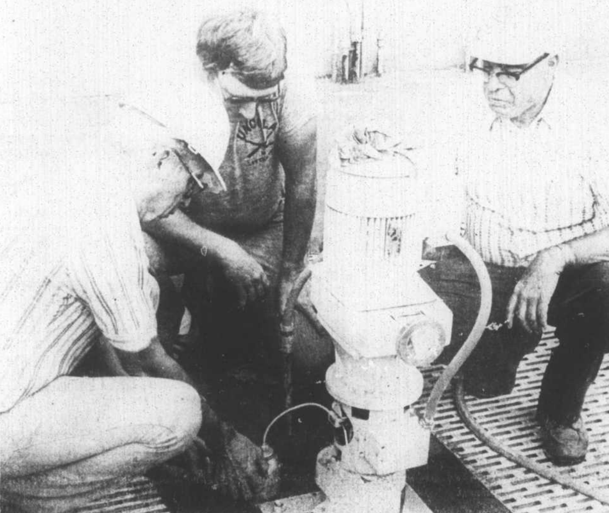
Workmen at the new $5 million sewage treatment plant south of Warrenton are shown working on an agitator which was flooded when the water level rose at the plant. The agitator, used to collect grit passing through sewer lines, is one of numerous items which are submerged periodically at the
