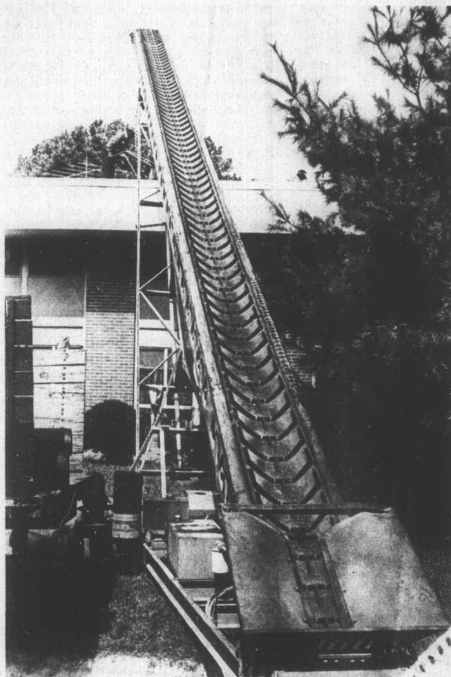
Workers from Pioneer Roofing Co. in Raleigh hope that good weather will enable them to finish putting a new roof on Mariam Boyd Elementary School within the next two weeks. The project, which began Monday, was needed to repair leaks and will cost approximately $49,000. (Staff Photo)
