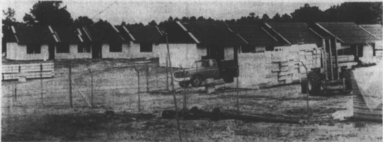
Construction continues on the 50-unit Pines Apartment complex on U. S. 1 north of Norlina adjacent to Northside School. Ruffin Woody Associates, Inc. of Roxboro, developers of the project, anticipate that it will be ready for occupancy next spring at a total
