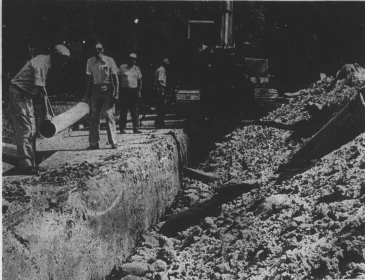
Town officials lent a helping hand in replacing 1,200 feet of sewer pipe on South Main Street in Warrenton last weekend in an effort to keep costs to a minimum. Shown above at the project site are
