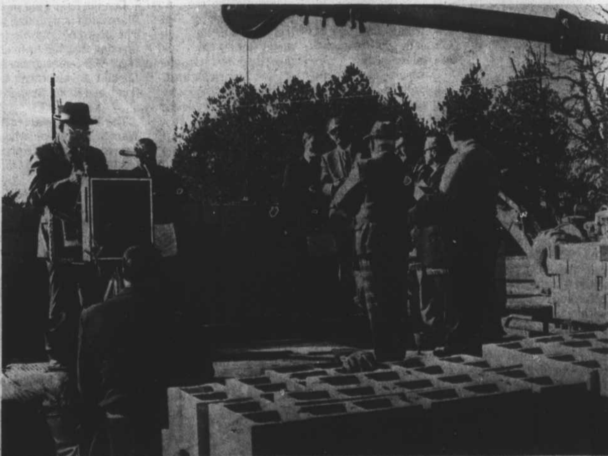
Members of Francis S. Packard Masonic Lodge of Norlina watched last Wednesday as the cornerstone was lowered in place at the lodge site on One Road. Cecil J. Liverman, (left), grand master of the
