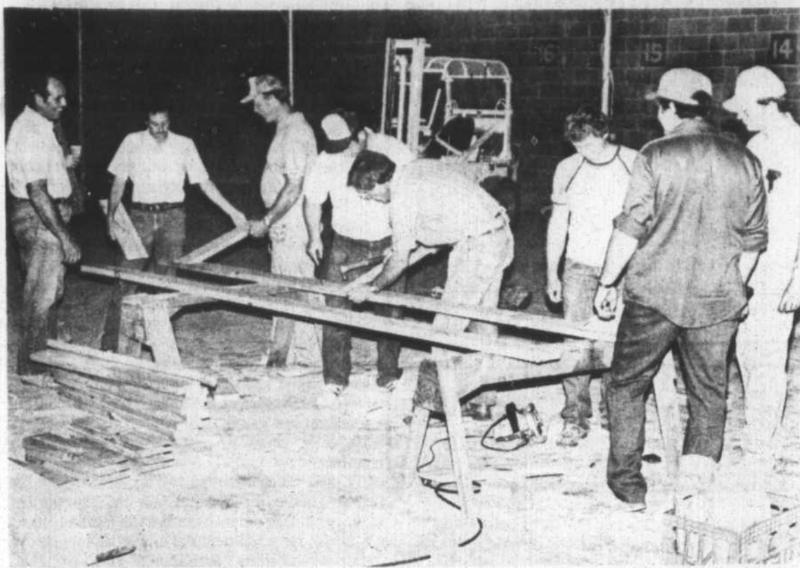
Afton rural firemen shed their firefighting gear to put carpentry skills to work rebuilding the stage for their annual moneymaking project, Hee-Haw,
