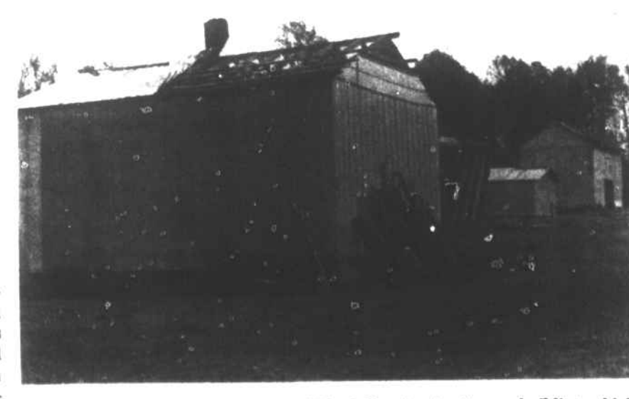
Pictured above is Oine resident Hubert Vaughan's storage building which was shifted from its rock foundation during an apparent tornado which swept through the area Sunday evening.
