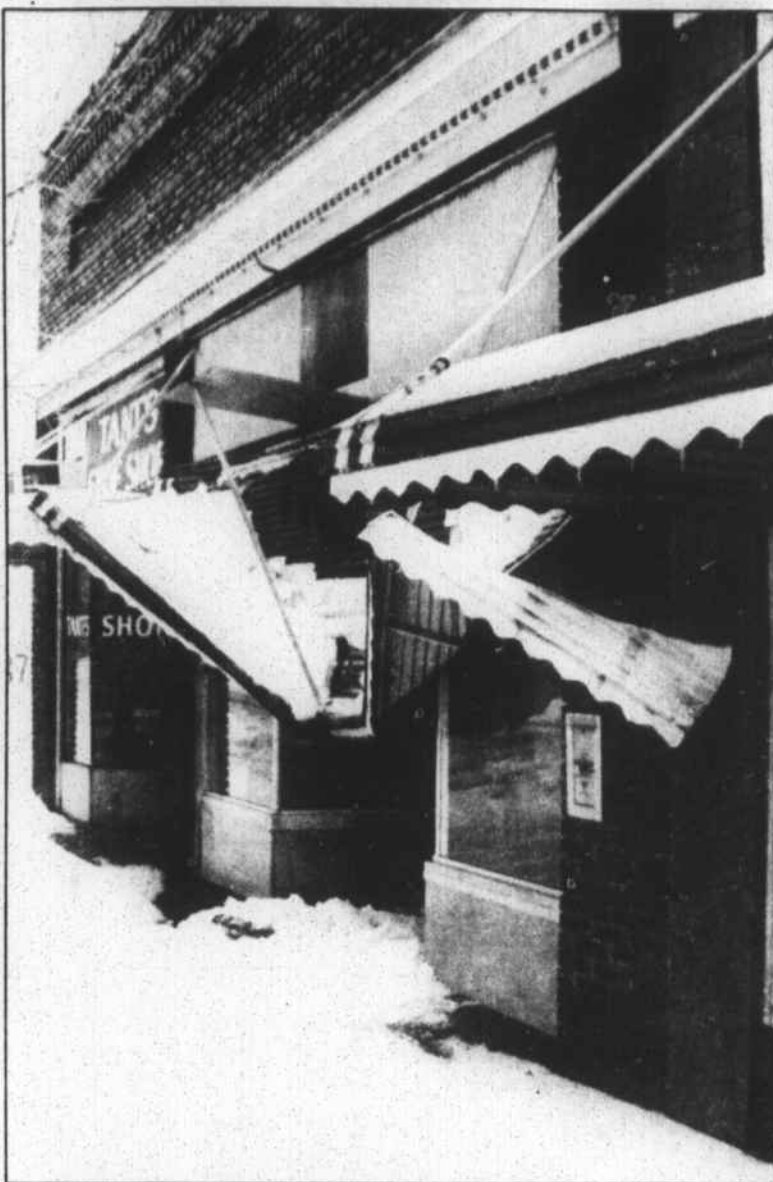
Citizens Insurance and Bonding Company's awning folded under the weight of more than three inches of sleet which started falling Monday and continued into Tuesday. (Staff Photo by Dianne T. Rodwell)
