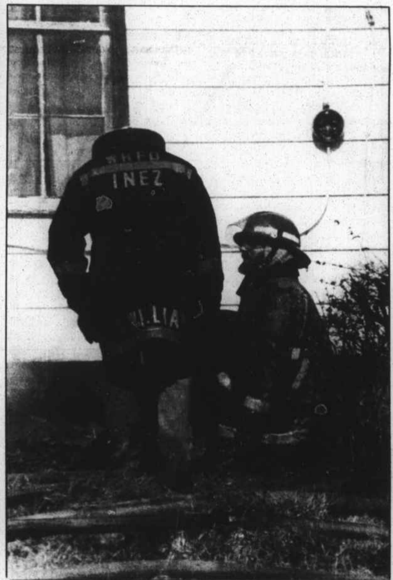
After knocking a hole in the foundation of the burning dwelling, Fireman George Alston (standing) of the Inez department and Rich Knisely of the Warrenton Rural department prepare to attack the blaze from underneath the house.
