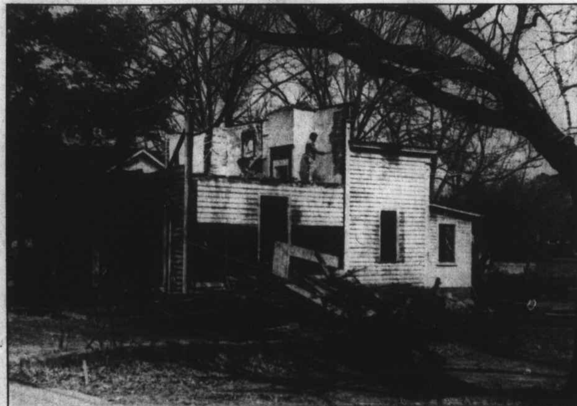
Timber by timber, workmen dismantle one of the town's houses of the 1800's, this one on the Ridgeway Street parcel purchased in 1984 by the Warrenton Baptist Church whose parsonage adjoins the property. This was not the first time the dwelling had fallen into Baptist hands, according to Lizzie Wilson Montgomery's "Sketches of Old Warrenton." It was purchased by the church during the pastorate of the Rev. James A. Mundy who
