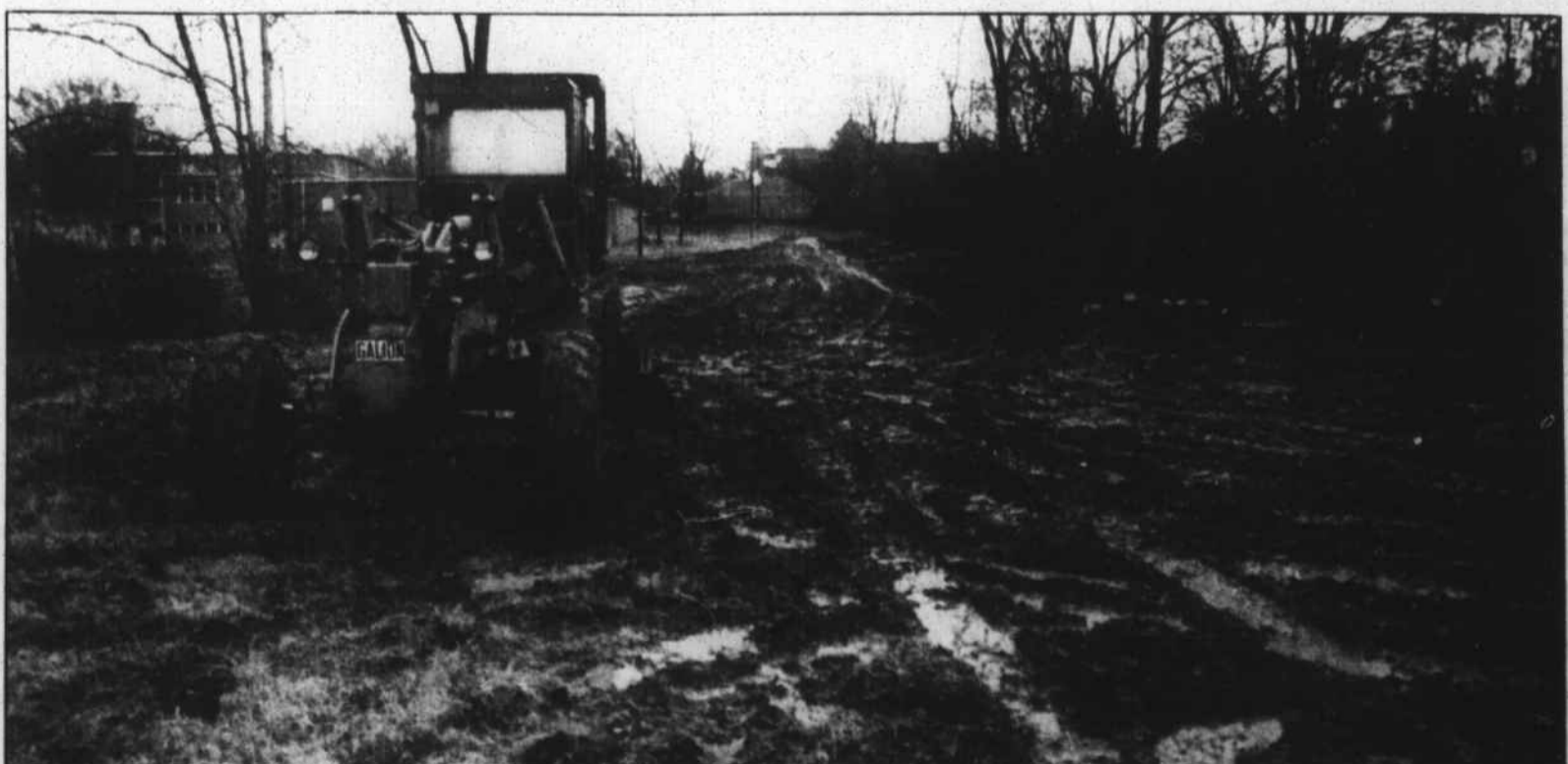
Work is under way on Vance Granville Community College's Warren County satellite facility being built on the John Graham Middle School campus here. Warren County Commissioners appropriated $70,000 to supplement the $400,000 in state funds for the project. Bids
