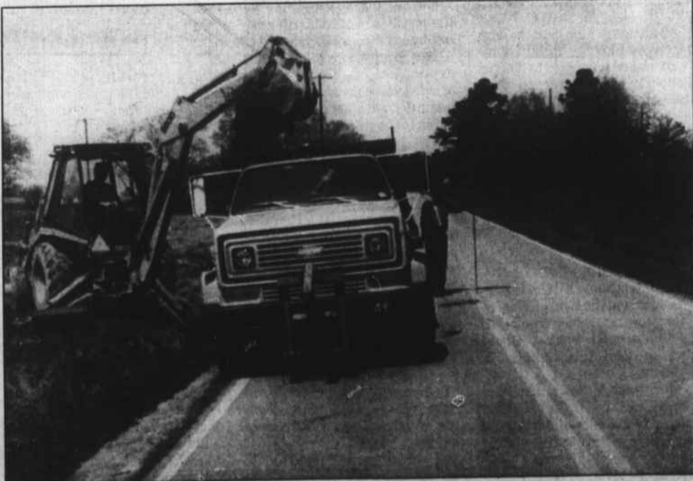
Long-time local DOT employee Gene Hudgins operates a backhoe in the work under way on the Warren Plains Road (SR 1305). A 2.1-mile stretch will be widened by two feet on each side. According to Donald Wall, DOT district engineer, the project will extend from the curbing and guttering section at the old depot and continue along North Main
