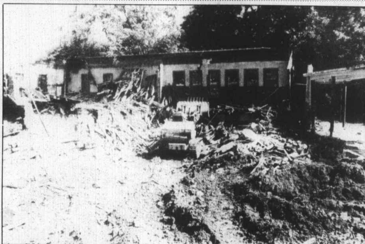
Demolition of the old brick building used for many years to house vocational classes, particularly agriculture classes, on the John Graham School campus began on Wednesday of last week. Paul Kearney, operator of a Warren County landscaping company, operates a
