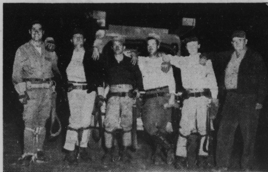
Ed Kitchings and his crew of construction workers, pictured above, worked Sundays and holidays as well as regular duty periods the past fall installing the local street lighting system. Members of the Carolina Power & Light Company group are, left to right, Dayton Parrish, Maylon Fuller, Henry Massey, Jeff Gordon, Johnnie Horton, and Foreman Kitchings.
