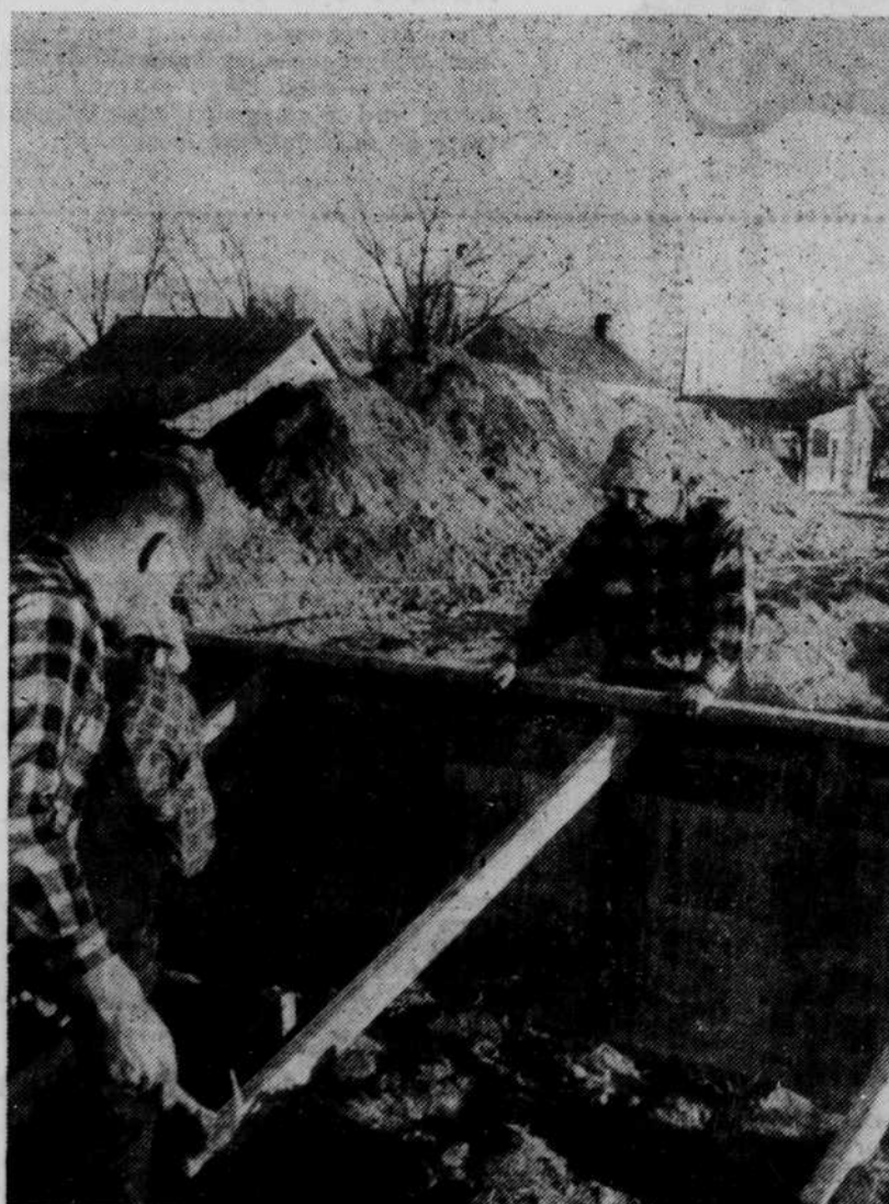
In the picture above excavation has been begun on the swimming pool for citizens of Zebulon and the community. Gordon Hammond of Wilmington, constructor, is seen looking down into the pool hole while a workman is hammering. The more than $30,000 project is expected to be completed by the summer.
