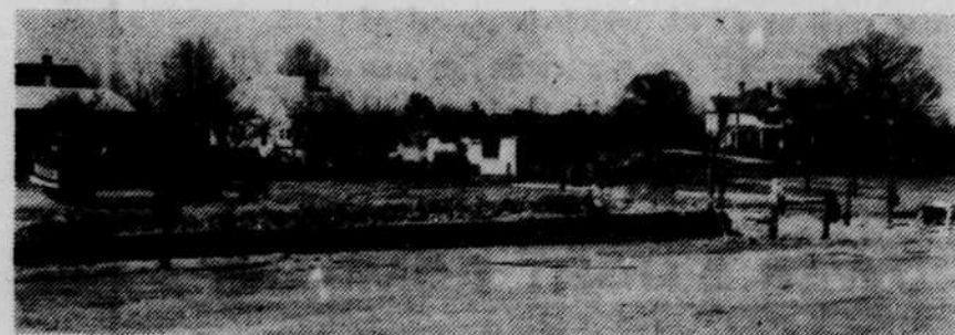
FIRST . . . The above scene shows workmen constructing the foundation of the first duplex apartment of the white low-cost housing development started here. Footings are being laid and work is proceeding on the project, which is located on the East end of Vance Street.
