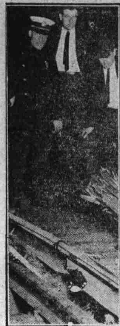
This section of a rail shows how near a train full of excursionists were to death when three bombs exploded under it at North Bergen, N. J. Had the rail separated the train would have been plunged over an embankment.
