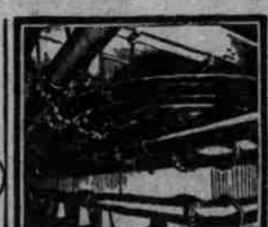
All steam, water and compressed air pipe-lines in the Goodyear plant are Crane materials
