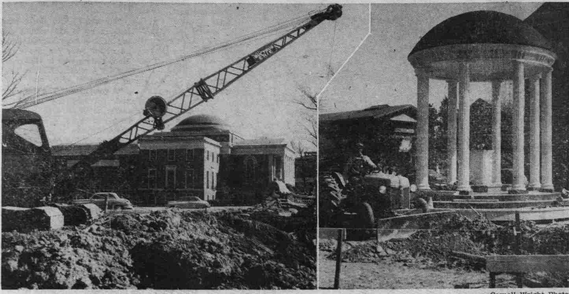
PROGRESS IS being made in what used to be the Planetarium parking lot and around the Old Well. Tractors, derricks and plain old shovels are rapidly making the parking lot into a bigger parking lot, with a garden in the middle; while over in front of South Building a formal garden is being laid out.
