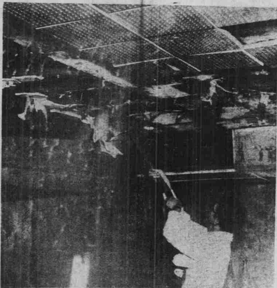
UNIDENTIFIED CHAPEL HILLIAN checking damage to basement ceiling at last night's fire at the KA House.
