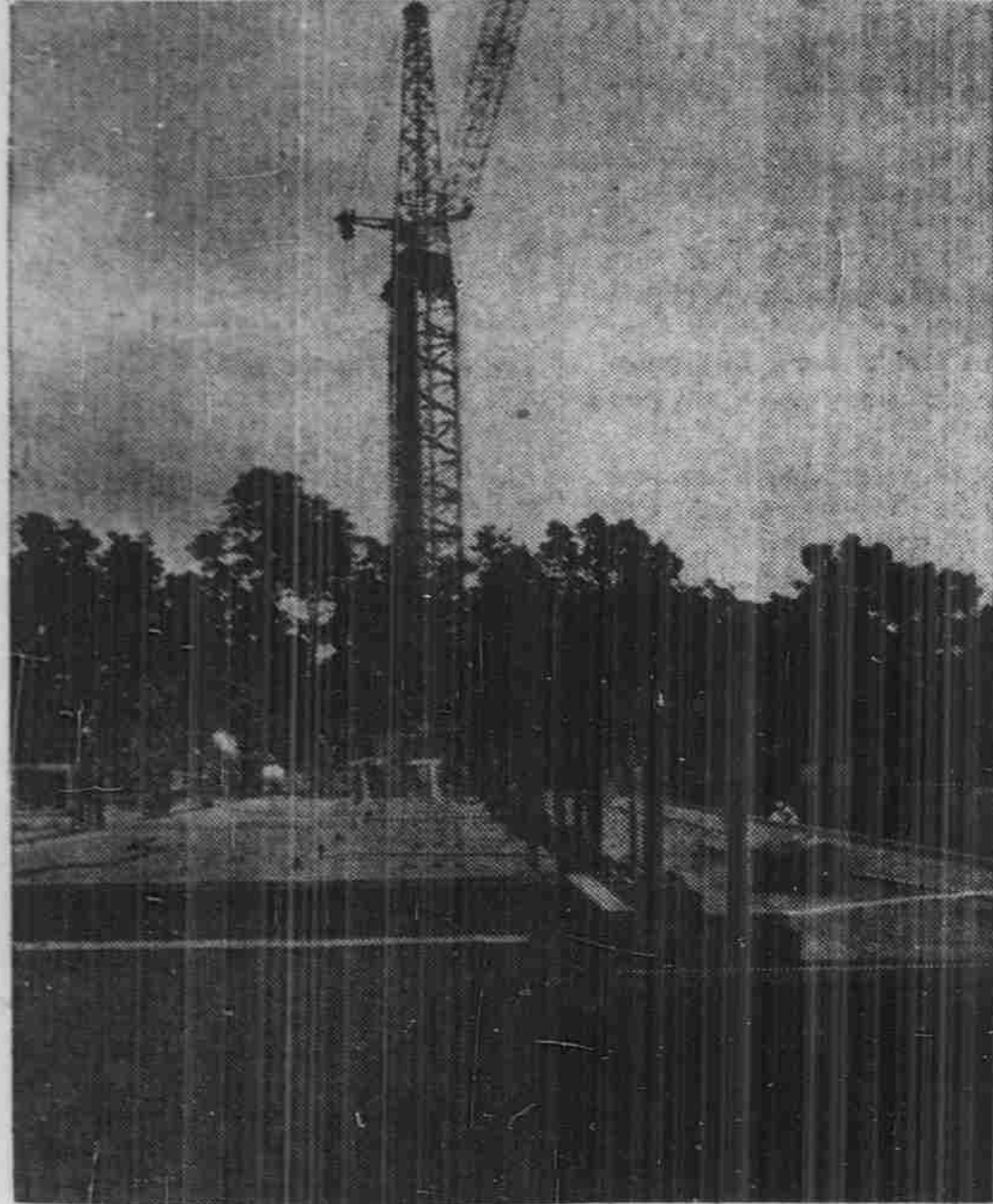
A 79-FOOT, electrically-operated crane lowers over the foundation of the new Burton Craige dormitory, which is supposed to be finished by December, said the work superintendent, "as a Christmas present for the students." The workers are presently engaged in pouring the cement for the first floor. Craige dormitory is being built in the woods past Parker-Teague-Avery, in the general direction of Columbia, S. C. (Photo by Jim Wallace).
