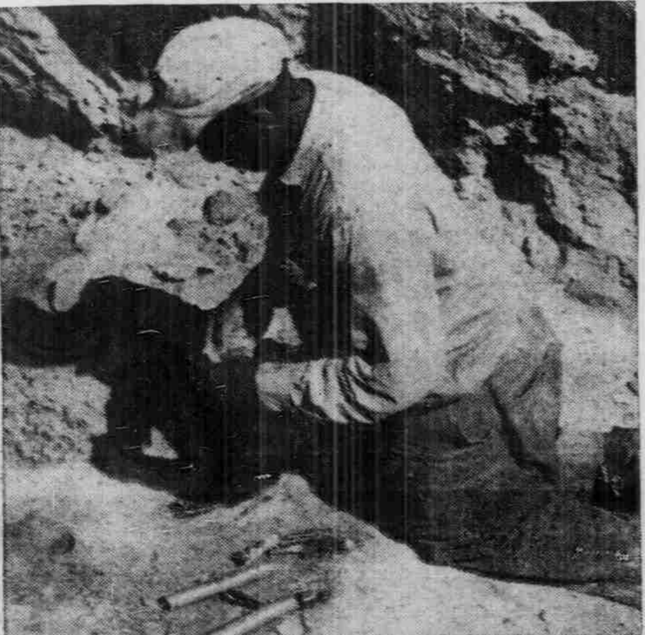
KENAN STADIUM—Construction workers digging the foundations for the addition to Kenan Stadium ran into a layer of rock last week and had to blast. Above, a workman places the dynamite.
