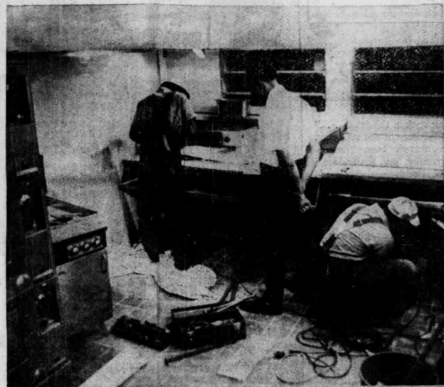
NEW KITCHEN — Workmen hurry to finish setting up the new cooking facilities in the Rat to replace those lost in a fire last summer. The Rat will be open again on Monday.
