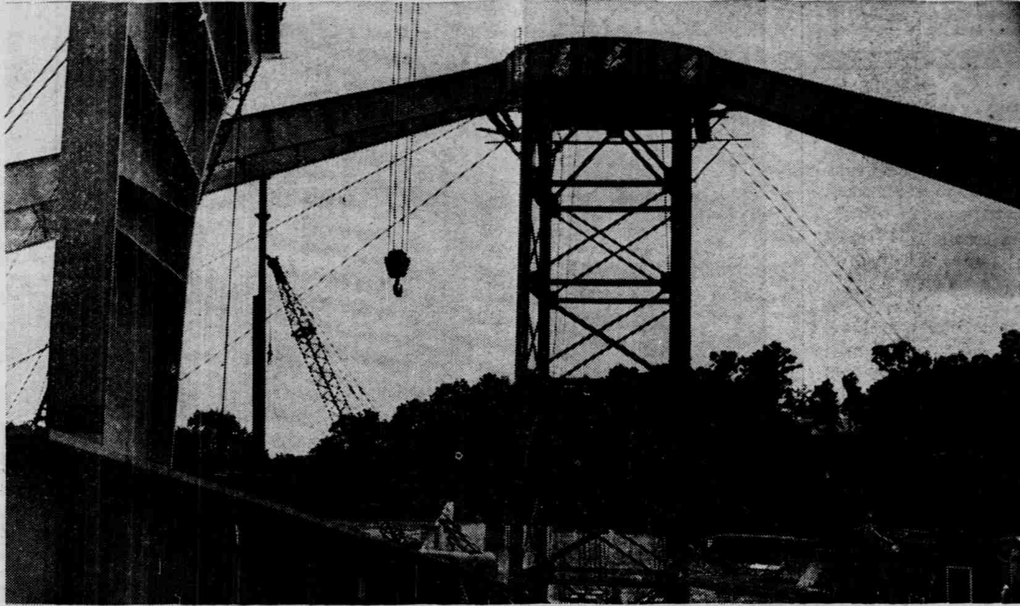
UP SHE GOES!! Construction on UNC's new annex to Woollen Gym is well under way. The girders, like the one above, will radiate from the center hub which alone weighs sixteen tons. The steel girder in this picture is 123 feet, which is not the biggest the gym will have.
