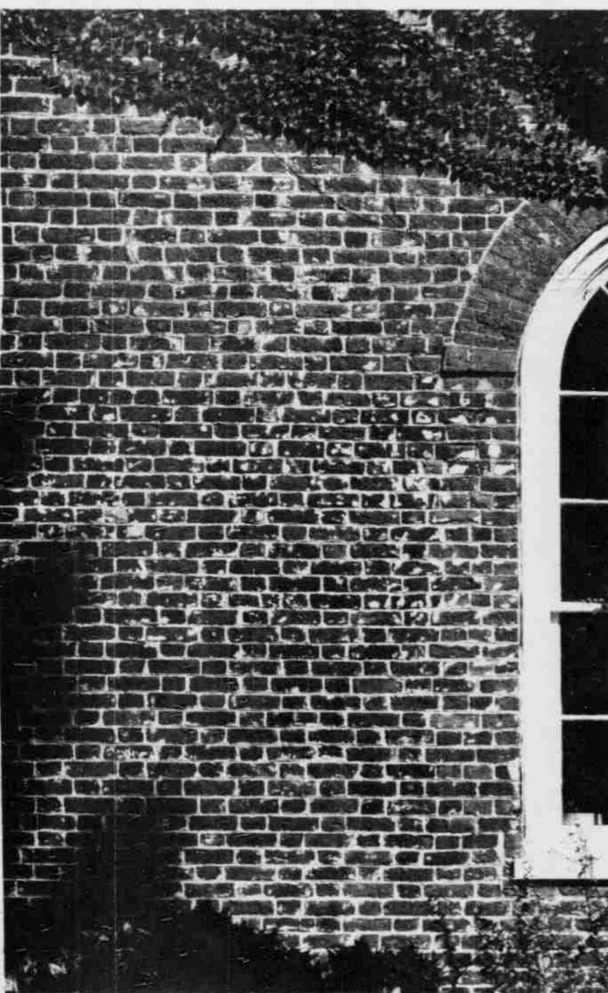
PERSON HALL TODAY, a detail from the wall which faces Old West. The wash has been removed revealing the 1795 wall laid in Flemish bond, a shimmering example of "colonial" brickwork.
