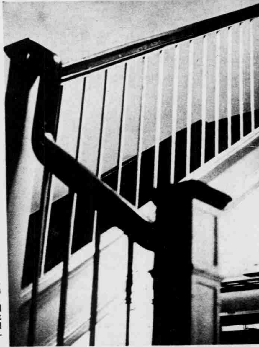
THE METAL STRIPPING on the edges of Spencer's old wing stairs, shown above, are worn to the point that they are slick. Such dangers in girl's dorms are being acted on by the Residence Hall Improvement Committee.—DTH Photo By Andy Myers
